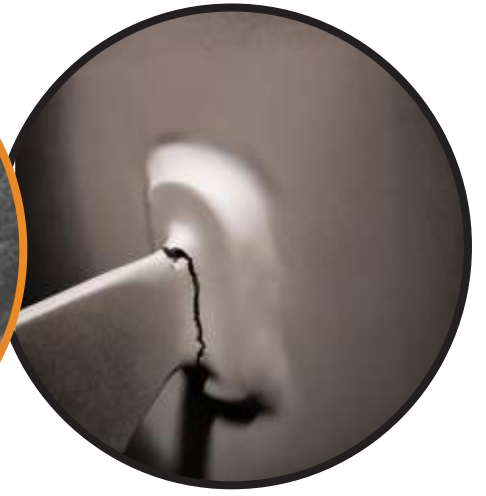
Non-compliant boss welding
